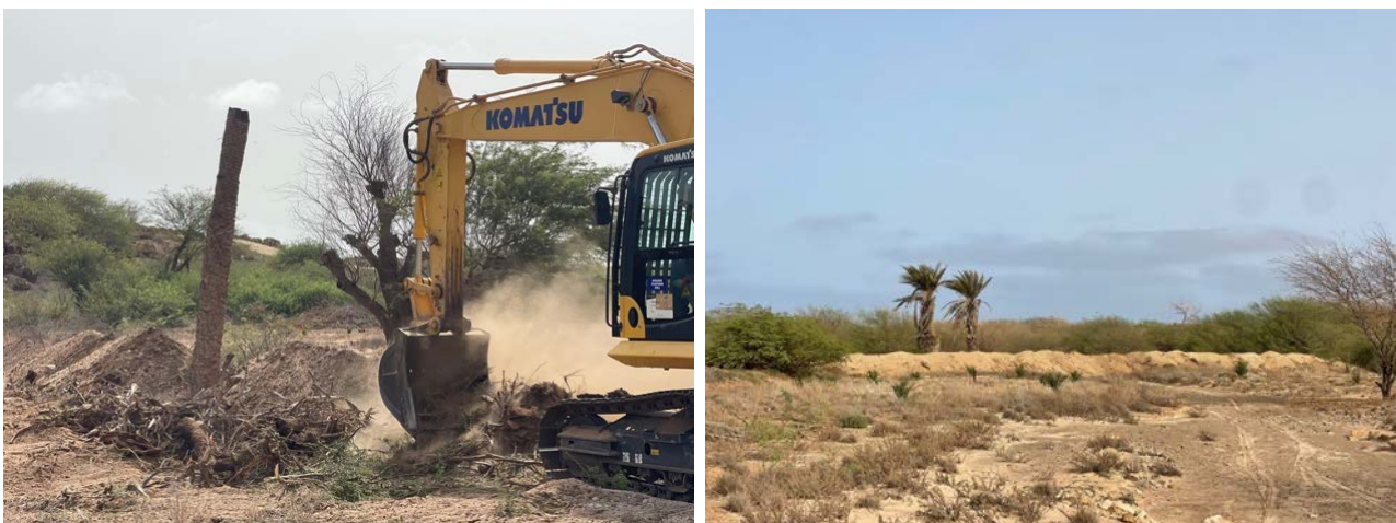
Figure 8 – Thanks to the collaboration with a construction company, a bulldozer was offered to unroot acacia trees (left) and to build a dam to retain or slow down rainwater and, therefore, decrease erosion and favour water absorption.
