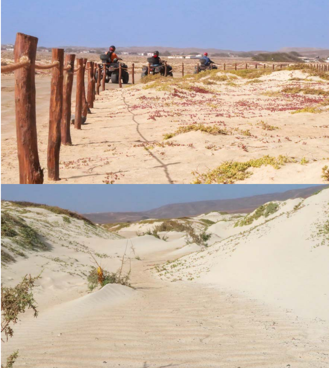
Figure 13 – Over 1,25 km of Protected Area path was fenced to stop vehicles driving on important foredunes (top). This was done using the acacia wood obtained during their pruning and felling from the palm trees oases. Some paths that used to be used regularly by pick-up drivers and quadbike excursions are being restored after fencing them off and planting new tamarisks (bottom).
