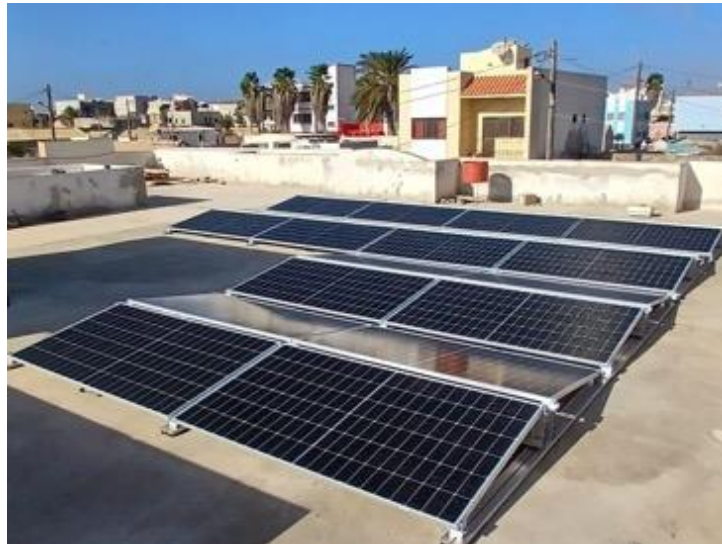
Figure 25 – Solar panels installed on the roof of the Association of Fishers of Palmeira.
